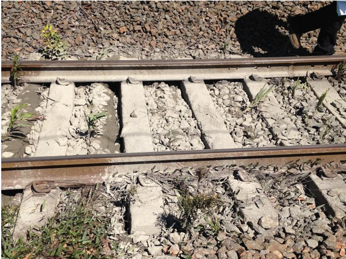
Fig. 1 Mud-holes occur when the ballast becomes contaminated (or fouled) with fine materials.
