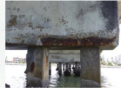
Deterioration of RC structures
