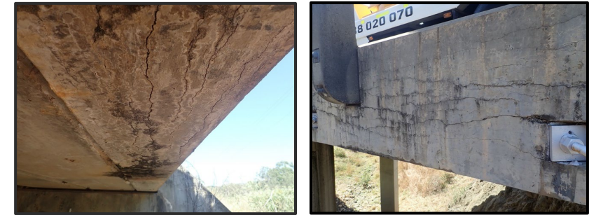
Original Inspection Photos Taken from ASR Affected Bridges in Queensland
