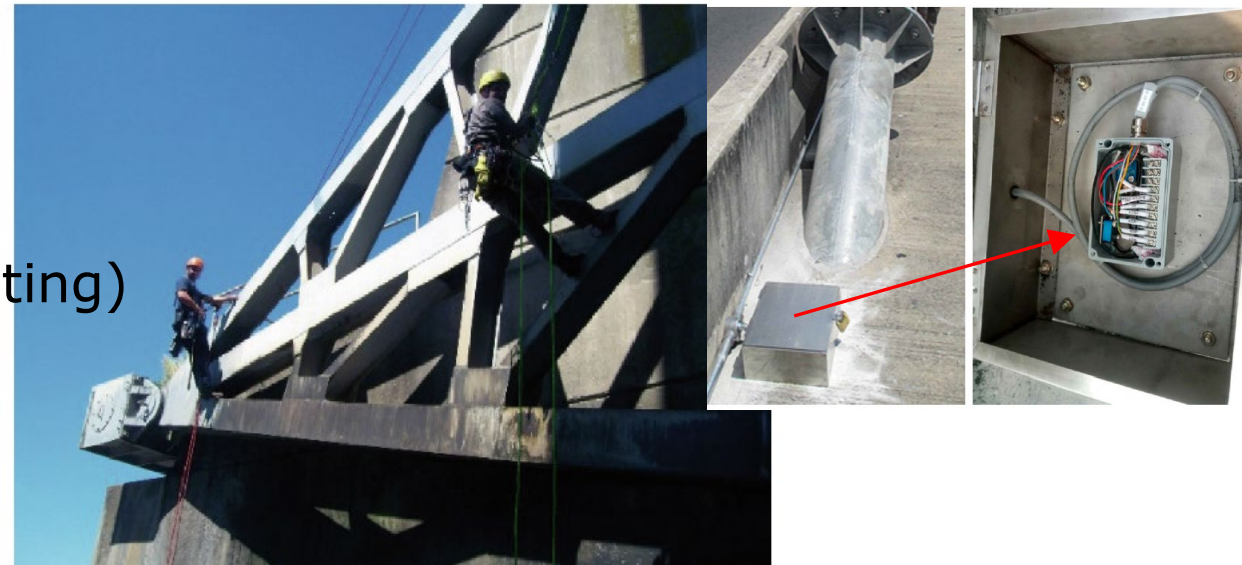
Inspectors from the US Army Corps of Engineers rappel down a Tainter gate to inspect for surface damage [4] (in Spencer 2019)
