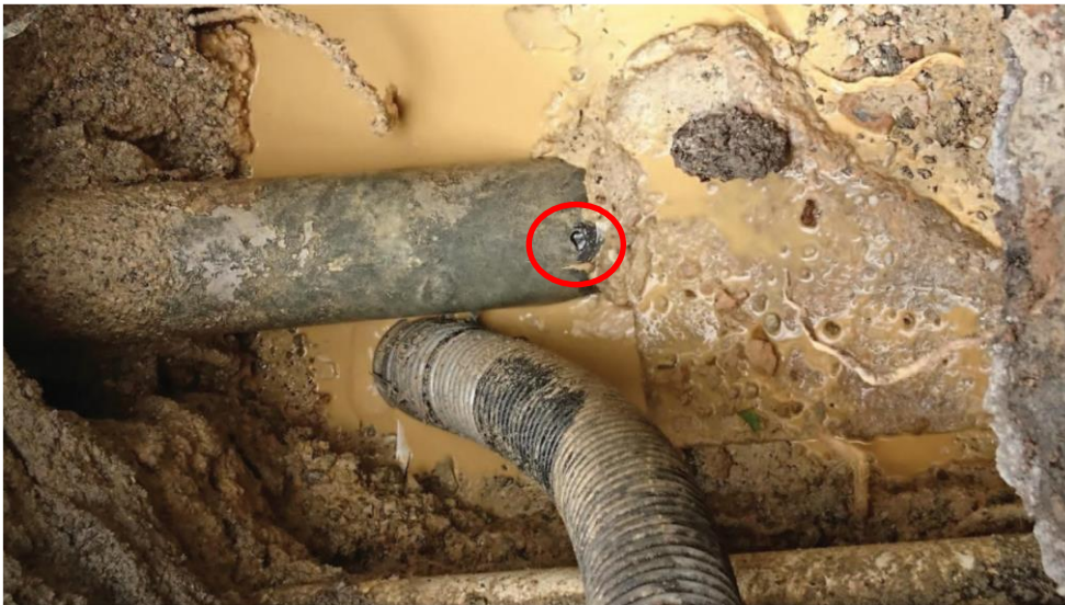
Figure 5. A circular crack (thumb sized hole, highlighted in the red circle) detected on a 150 mm mild steel cement lined (MSCL) pipe [adapted from Zhang et al. (2022a)].
