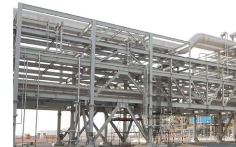
Petrochemical Pipe Rack (copyright by hardhatengineer.com)
